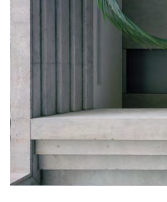
D - OFF FORM CONCRETE DULUX ASWATERED TO 'MAY GRAY' ELIZABETH STREET - CANDALPAS ASSOCIATES
